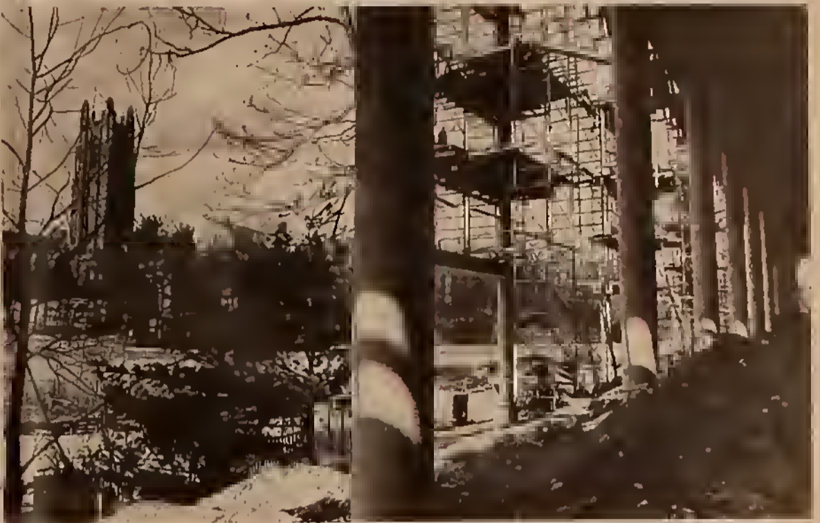
Construction on Science Center, scheduled to be completed by 1976, forges ahead as a result of recent good weather. photo by Sasha Norkin '75
